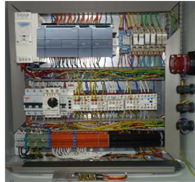
Figure 6. Electrical cubicle of water well
