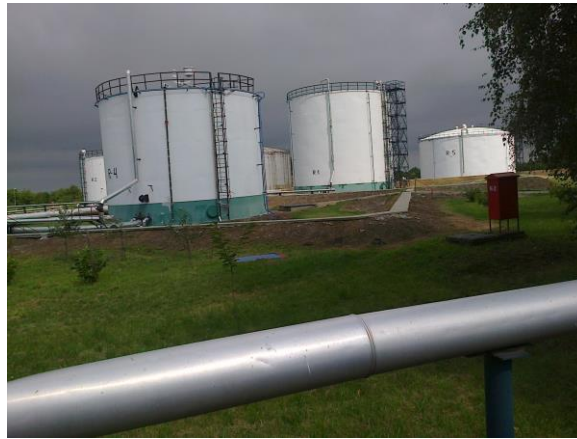
Figure 3. The appearance of the oil collecting station
