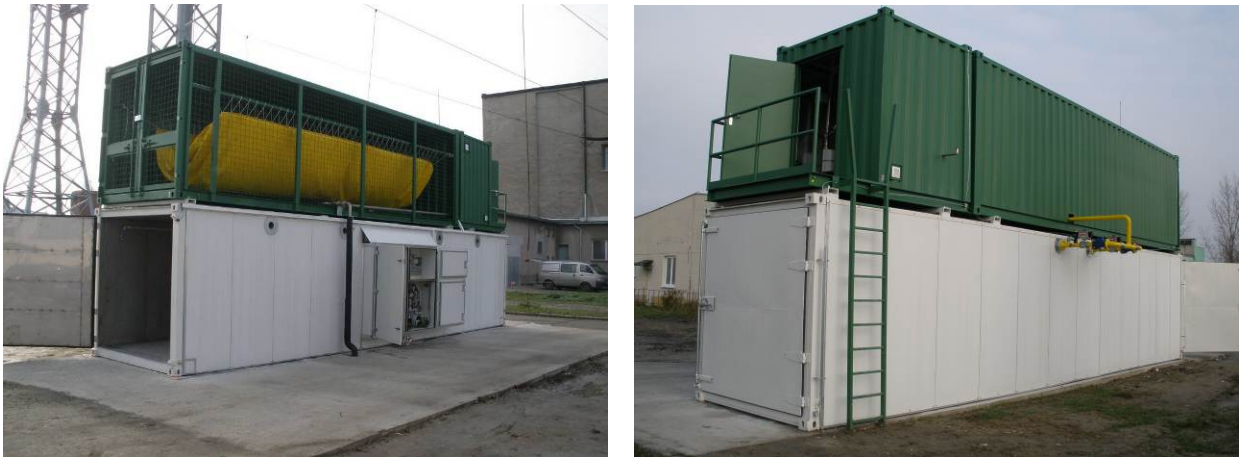
Figure 6. Dry fermentation container facility
